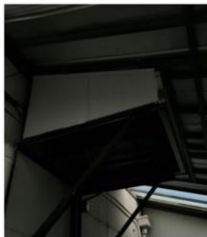
Panel y Filtro interior
