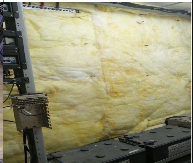
Lana mineral instalada
