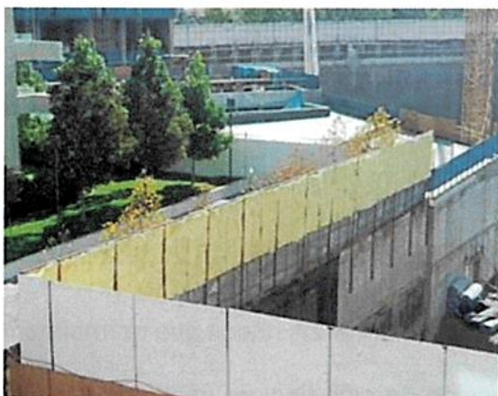
Cierre perimetral sector receptor Ad3
