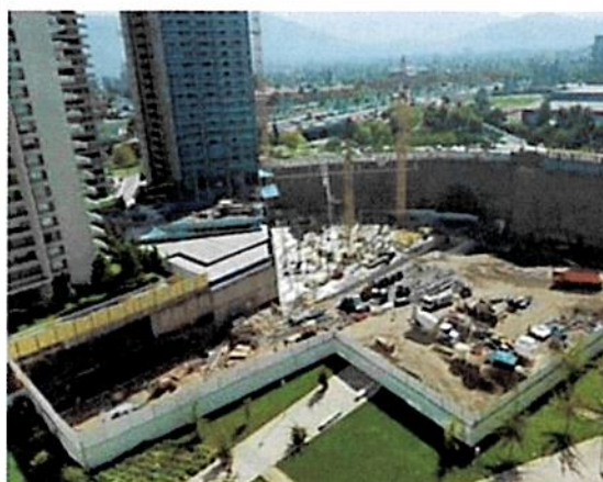
Cierre perimetral sector receptor Ad3
